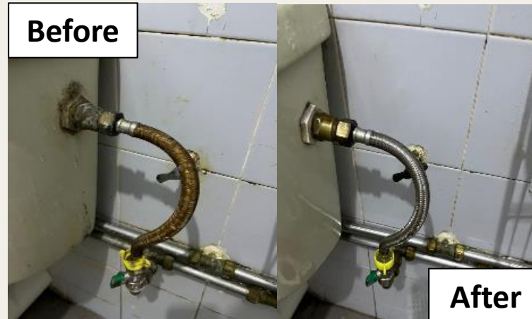
Washroom Stain Surface Cleaning
